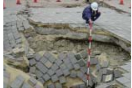
Damage from the 2005 Fukuoka Prefecture Western Offshore Earthquake
