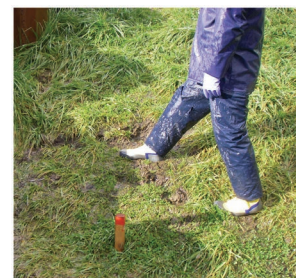
写真-2 のり尻部の泥濁化 Photo 2 Muddy situation with seepage water at the foot of slope
