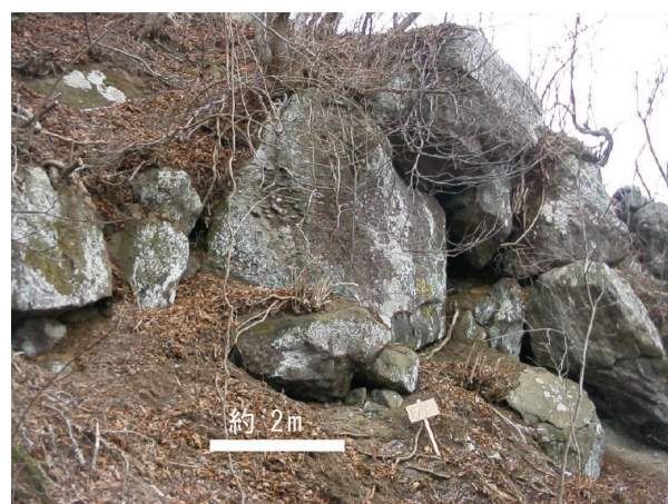
写真-4 E地区 中間斜面の浮石 Photo 4 Loose part of rocks in E area.
