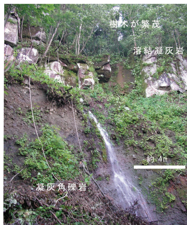
写真-3 D地区 湧水箇所の状況 Photo 3 Spring of ground water spring in D area.
