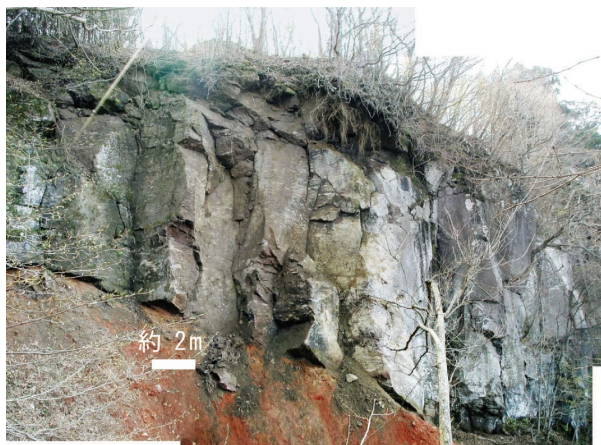
写真-1 E地区 溶結凝灰岩露頭 平成15年5月1日の落石発生地点 Photo 1 Outcrop of welded tuff in E area. (The rock fall has occurred in May 1, 2003.)
