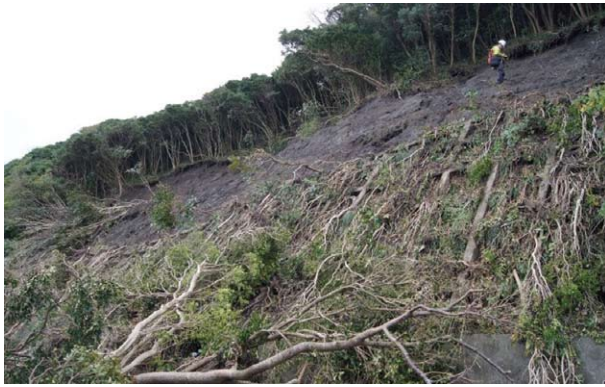
写真-2 のり枠上方の表層崩壊 (②地点) Photo 2 Slope collapse above slope crib (Site ②)
